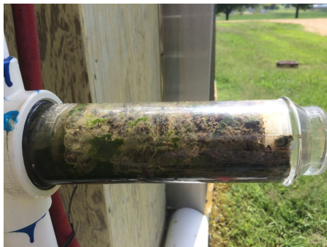
Figure 1. A clogged filter. Photo: Tom Tabler
