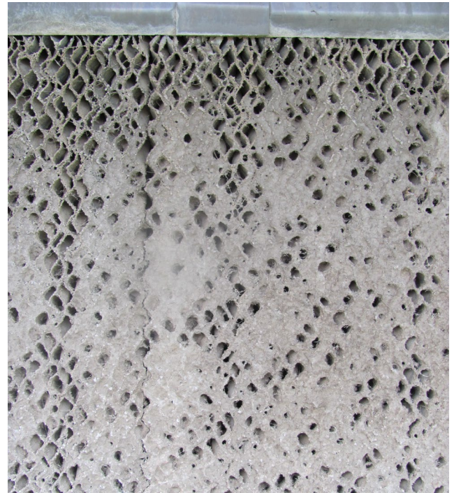
Figure 2. A clogged cool cell pad. Photo: Tom Tabler
