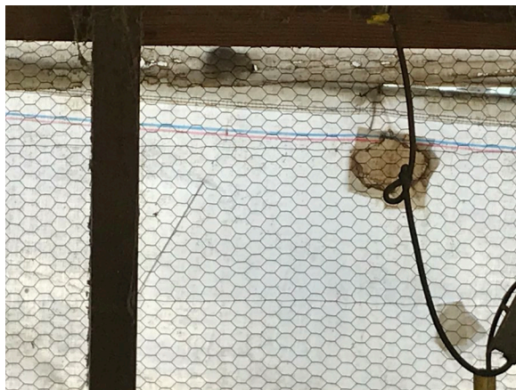
Figure 3: Rodent on top of roof
