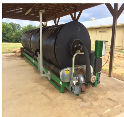
Figure 3. In-vessel rotary drum composting system.
