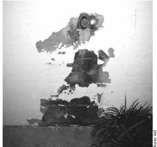
Figure 12. Faucets should be repaired before they cause this amount of damage. Moisture next to the foundation will attract termites.
