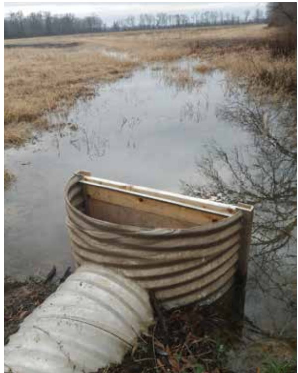
Fig 77a and b; Constructing a shallow dike across a flat field can enable you to provide excellent feeding and loafing areas for waterfowl. A water control structure allows the water level to be manipulated when fields are flooded. Top photo by Ryan Basinger; bottom photo by USDA-NRCS.
