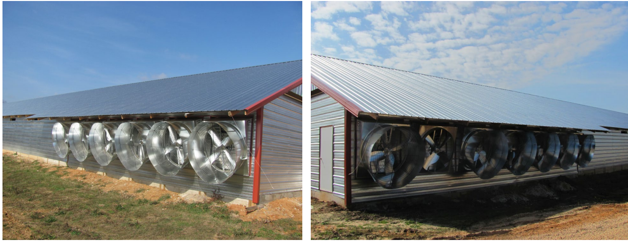
Figures 2 and 3 Fans must be in good condition to perform at their best. This requires inspection and routine maintenance, especially for minimum ventilation fans that work more than the rest.
