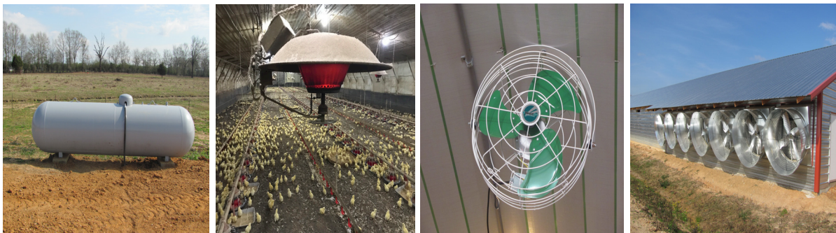
Figure 4a-d. Managing the transition to fall weather requires both heat and air flow to keep birds in their comfort zone.
